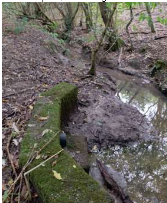
Old brick drainage works, still issuing water from the school
