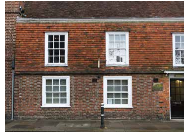
Façade cladding with clay hung tiles (upper storey) and bicolour brick (ground floor).
