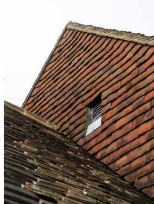
Details of a clay plaintile roof and a gable covered with hung clay tiles.
