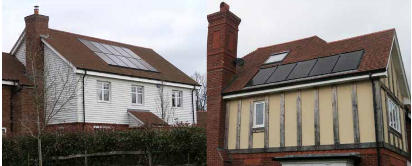
Figure 64: Solar panels on integrated into the structure and laid flush with the roof surface of newly built homes in Lingfield, Surrey.
